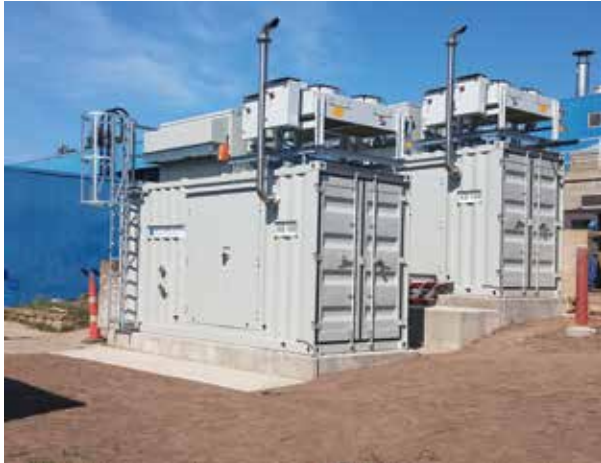
Twin KB 100 Biogas CHP Modules Pictured above
